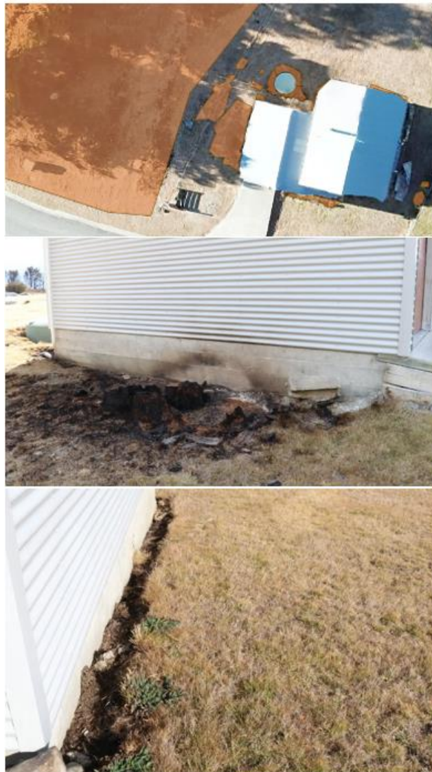
Figure 4. Post fire images of property C at Lake Ōhau. Area highlighted in brown in the top image shows where the fire burnt. The other images show significant burning of fuels up against the house. Photos supplied by FENZ, (2024).
