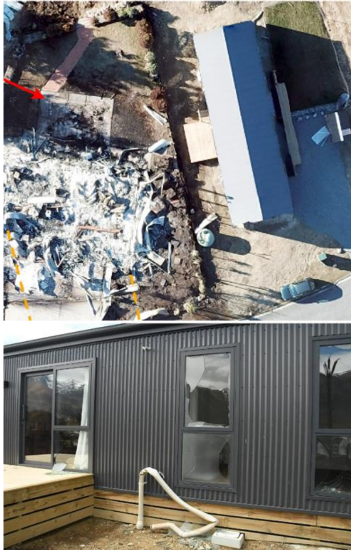
Figure 5. Post fire images of property D at Lake Ōhau with significant defensible space. The red arrow indicates the direction that the fire travelled in. Photos supplied by FENZ, (2024).
