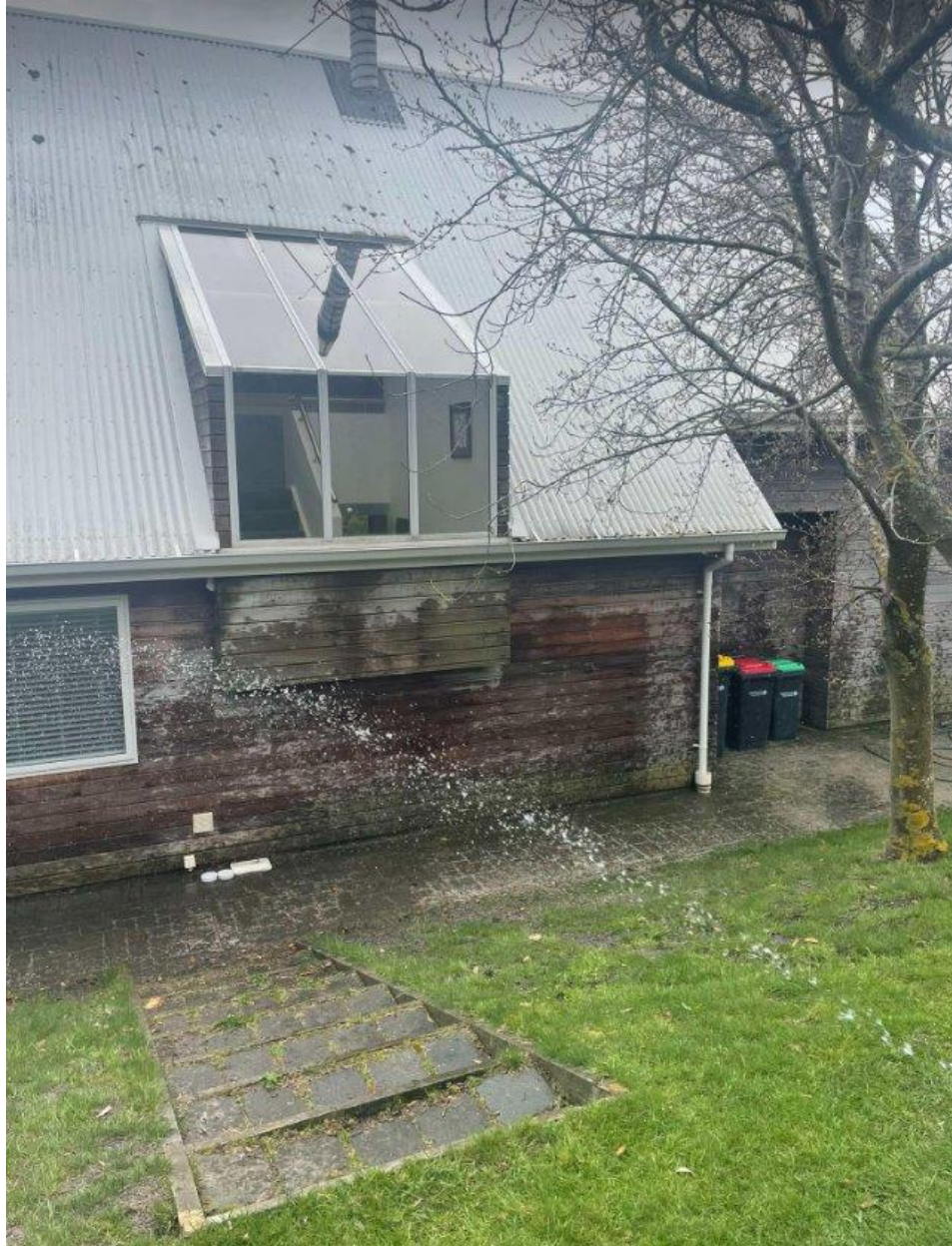
Figure 2. Sprinkler system on the rear of Property A on the Port Hills. Sprinklers could wet the wooden slats on the sides of the house to prevent them from burning in a fire.
